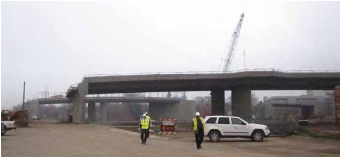
Construction of the Fifth and Sixth street bridges, linking the Railyards to downtown Sacramento.
